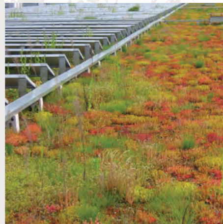
Extensive (limited substrate) Green Roof
