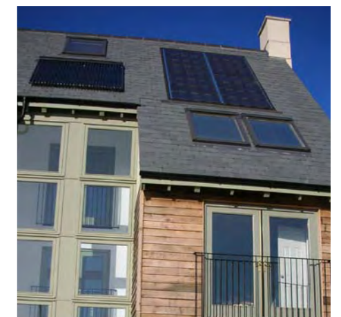
Photovoltaic and Solar Hot Water Panels
