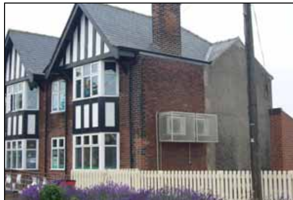
Air-condition units on a wall
