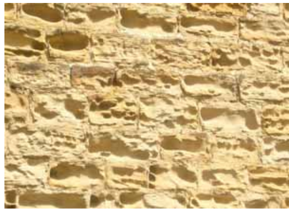
Eroded stone wall
