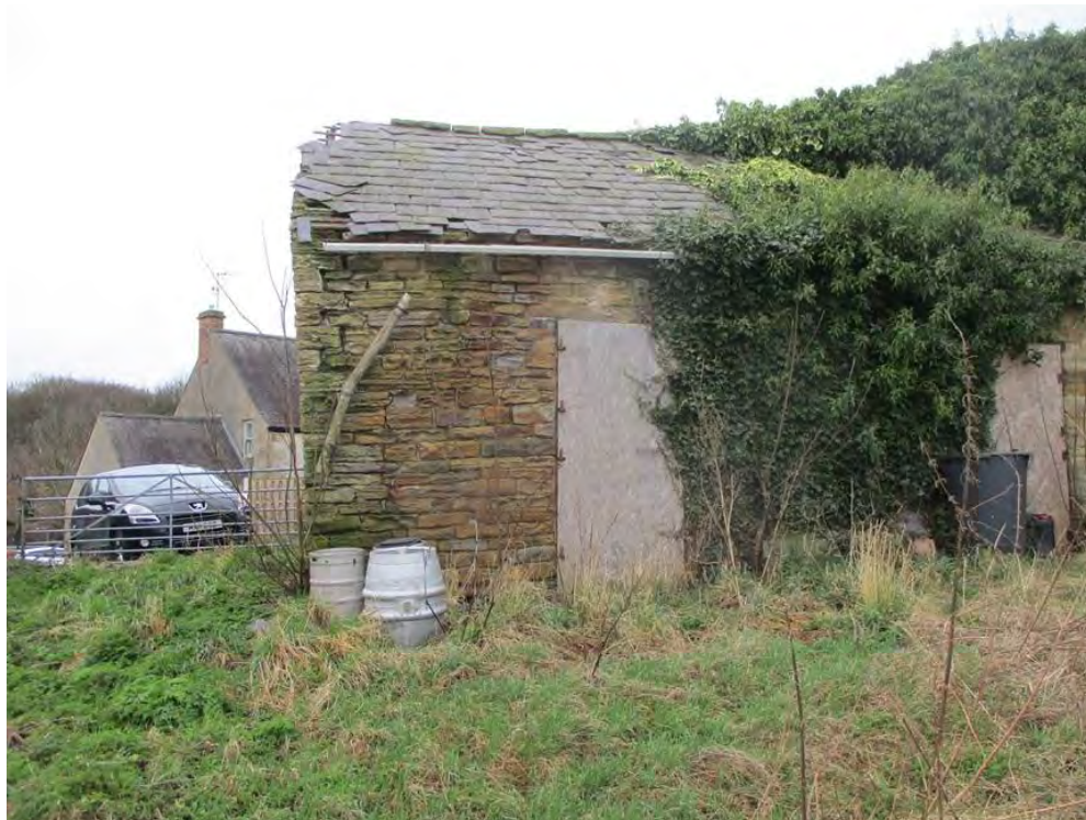
DILAPIDATED BUILDING BY ENTRANCE
