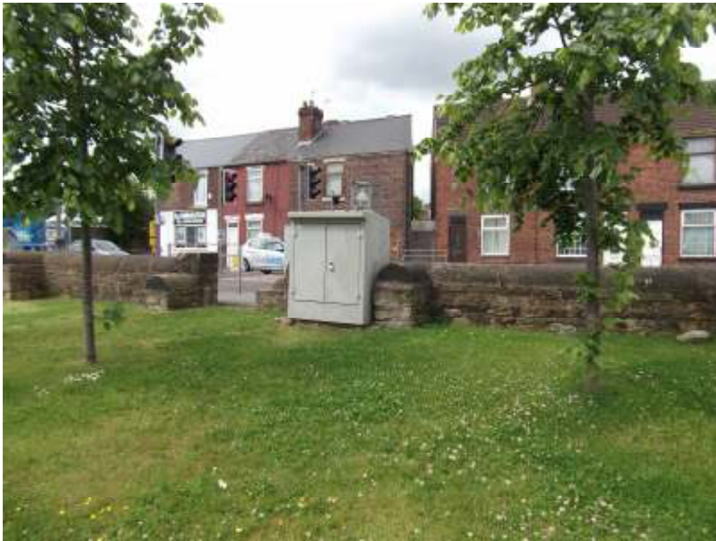
Figure D.6: Location of Sampling Head in Relation of the Affected Row of Terraced Housing on the Opposite Side of Sheffield Road
