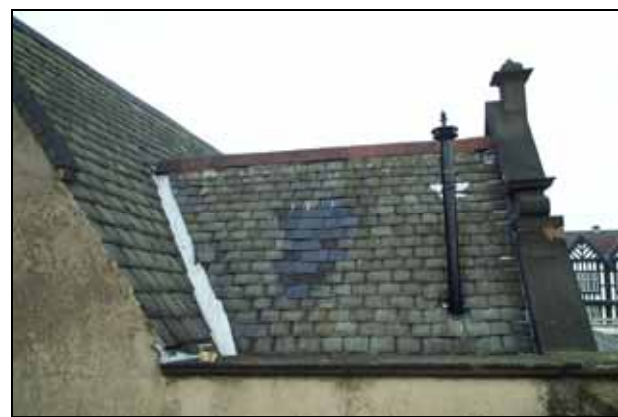
Poorly maintained roof
