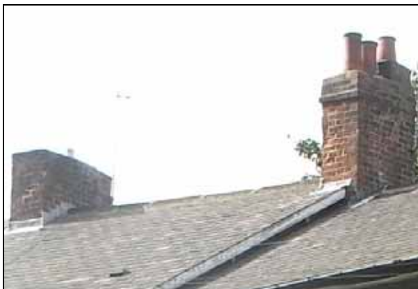
Loss of chimney pots - left
