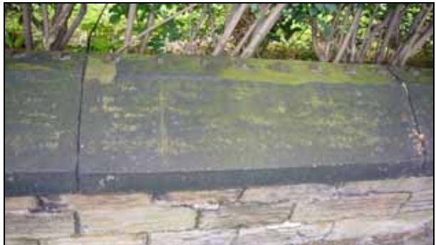
Stone coping showing removed railings holes
