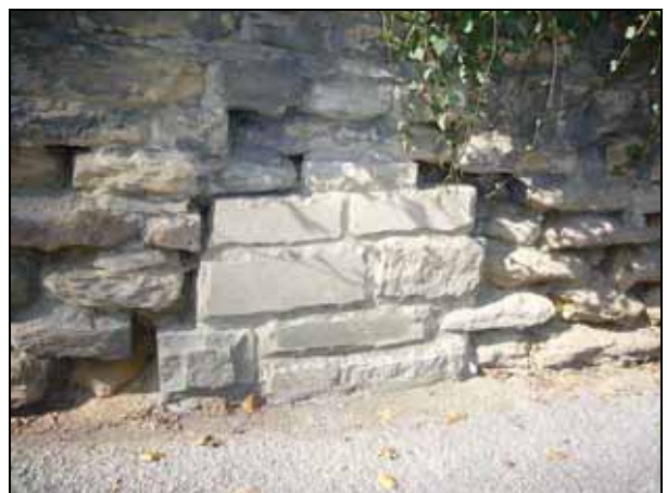
Inappropriate repair of traditional stone walls
