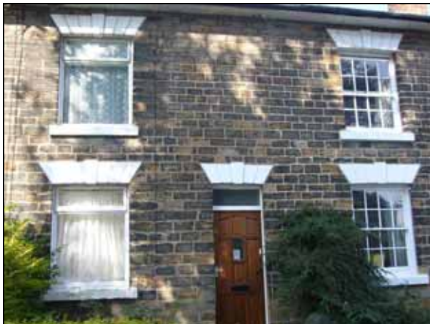
Inappropriate window replacements
