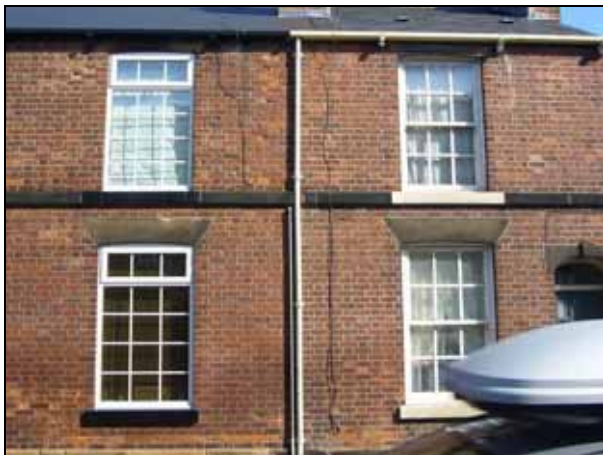
Non-matching uPVC replacement window on the left
