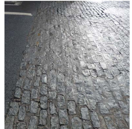
COBBLE RUMBLE STRIPS
